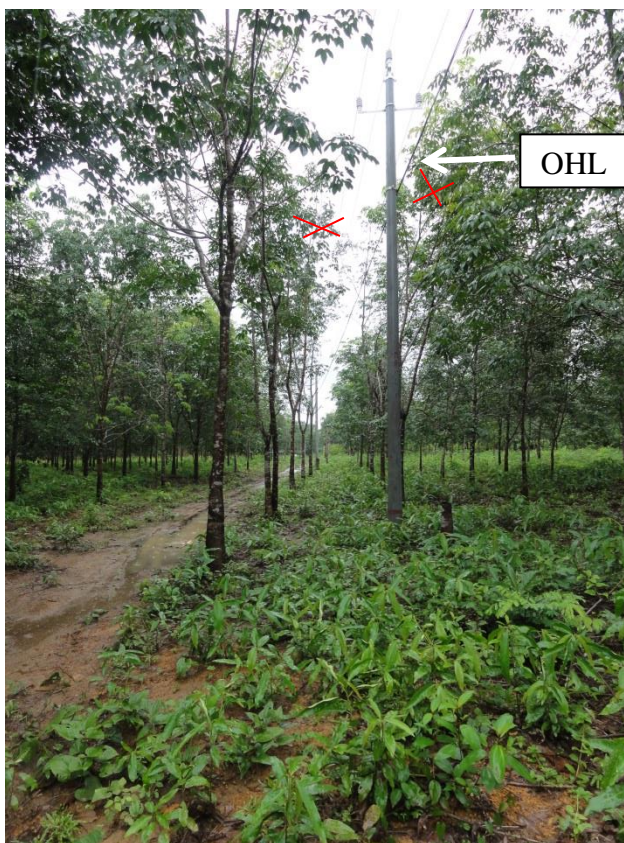
Figure 5-10: Line section where more branches of rubber trees have to be cut (red crosses).
