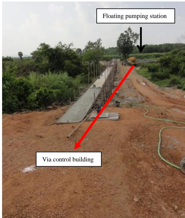
Figure 5-13: First pipe section from the pumping station to the control building (May 2017)
