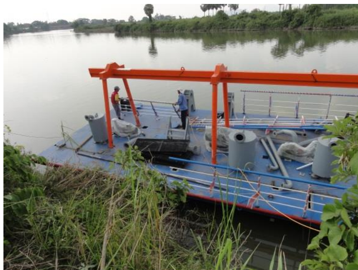
Figure 5-12: New floating pumping station (May 2017)
