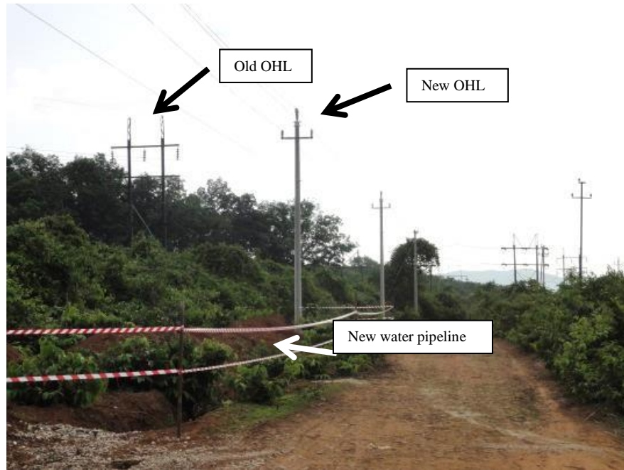
Figure 5-7: New water pipeline and new 6 kV OHL constructed between track and old OHL (May 2017)
